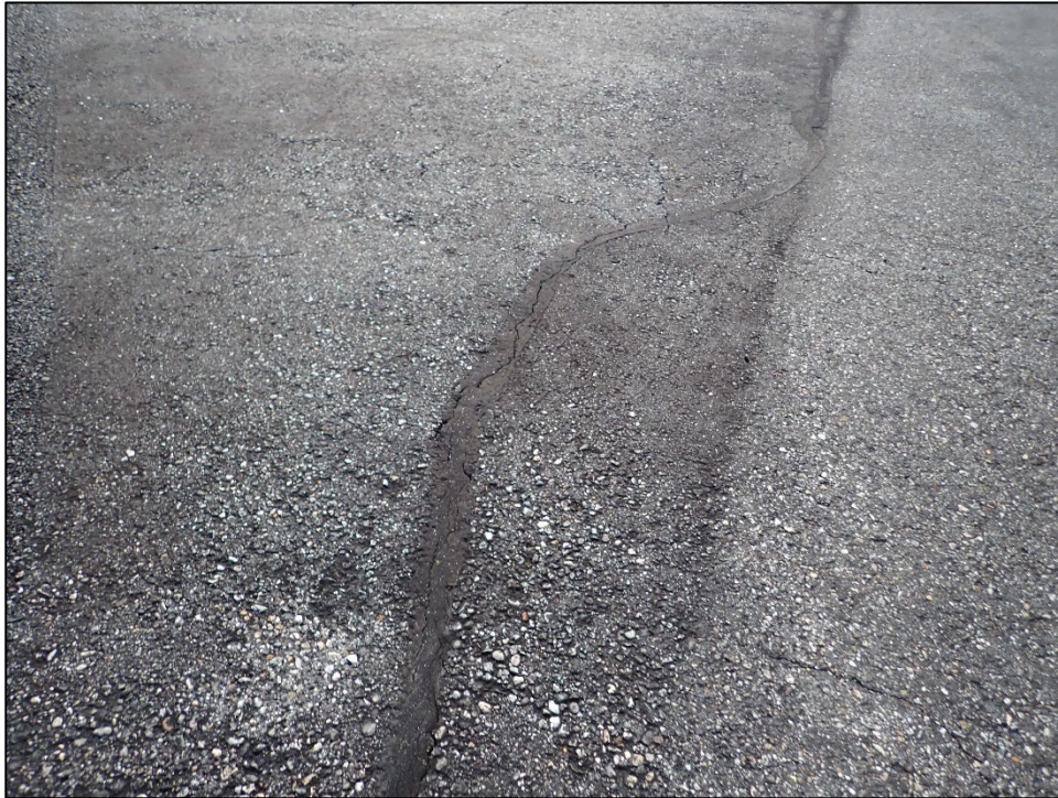
TW-02-02: L&T Cracking
