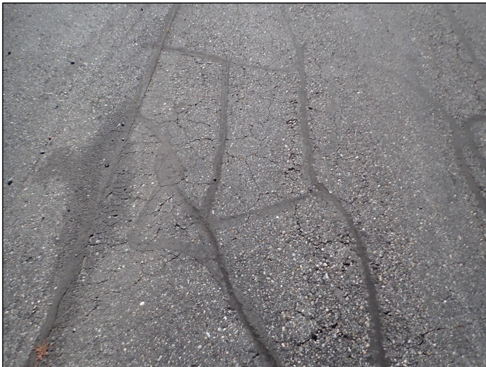
TW-02-07: Alligator Cracking
