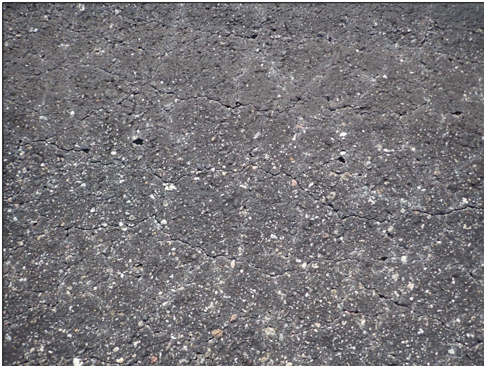
RW06-01-68: Alligator Cracking
