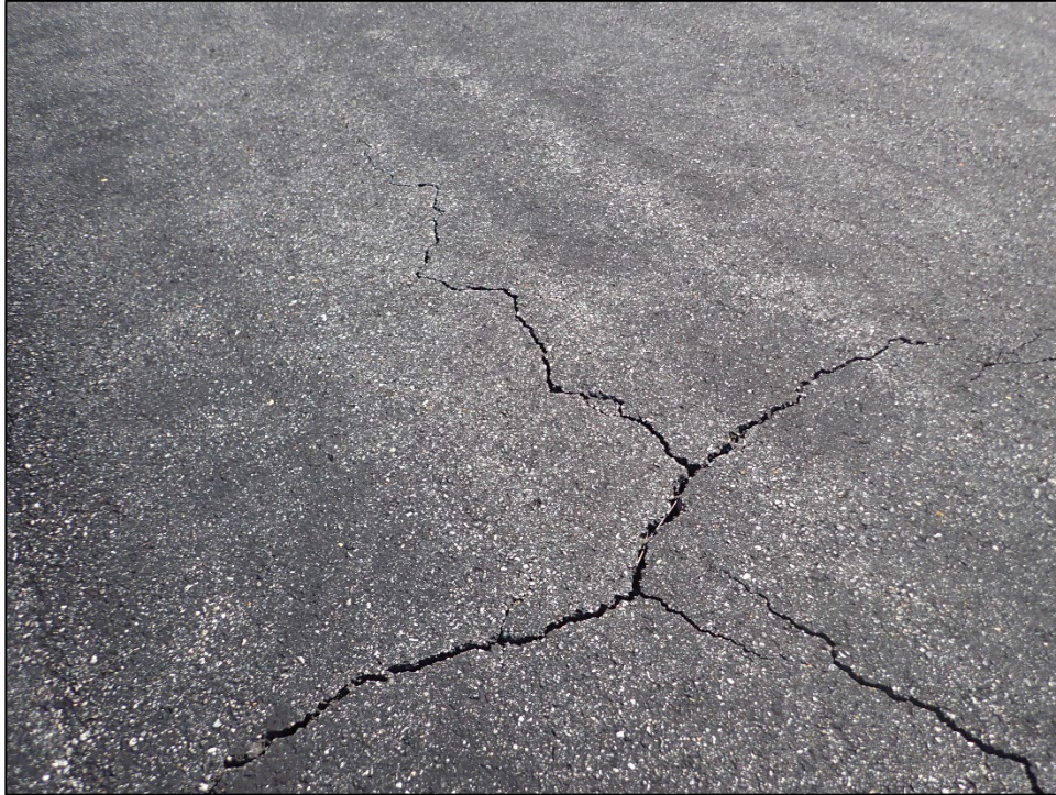
RW06-01-20: L&T Cracking
